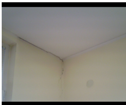
Fig. 12 – The problem of cracking of the wall (visual image).
