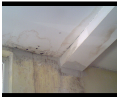
Fig. 9 – The infiltration of water and moisture problem (visual image).
