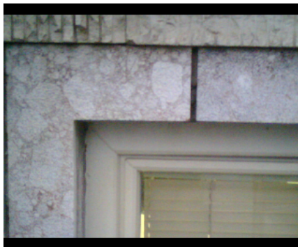
Fig. 6 – Poorly built and installed windows and insulation problem (visual image).
